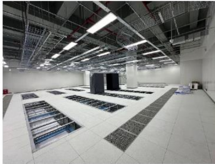
The front-end DAQ computer server room
