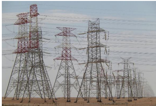
Electric power transmission
